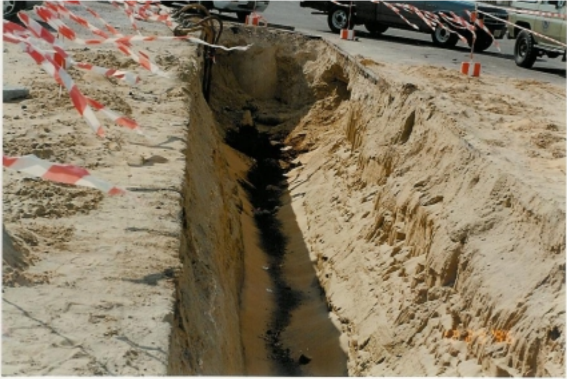
Plate 1.2 A photograph showing contaminated ground water and soil due to a leaking underground fuel storage tank in Dammam, Saudi Arabia (source Dr. Aiban, special collection)
