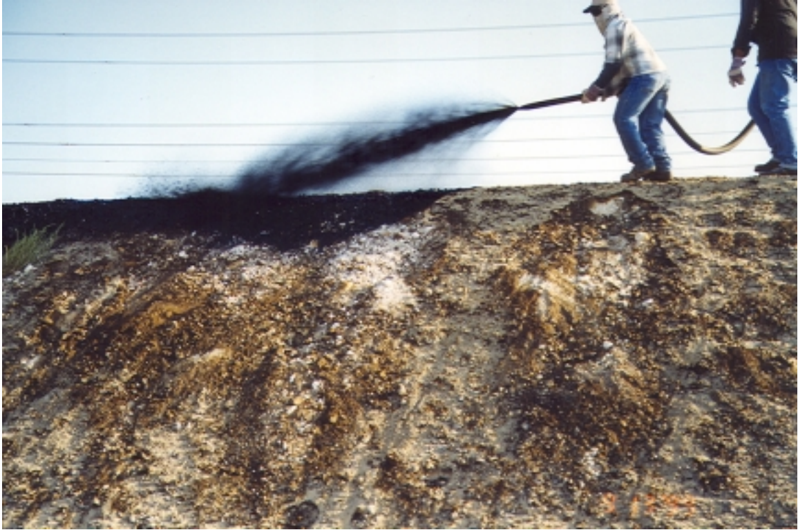
Plate 1.1 An example of crude oil spraying to stabilize the embankment near Dammam city (Aiban 1998)
