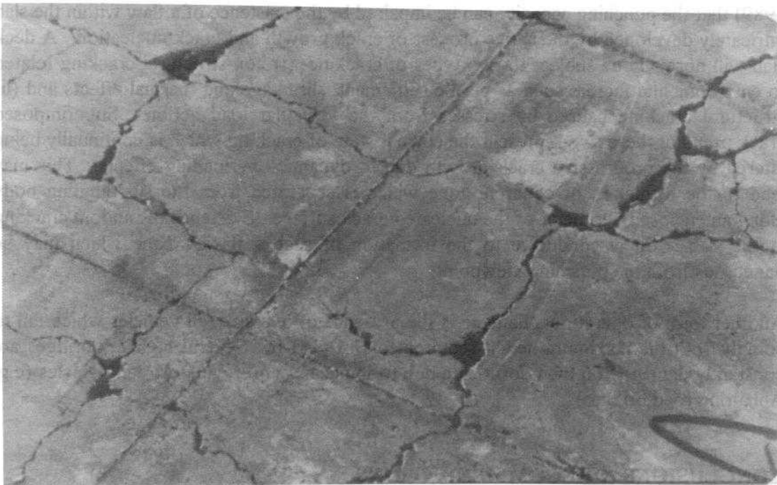
Plate 5. Extensive cracking of the deck slab
