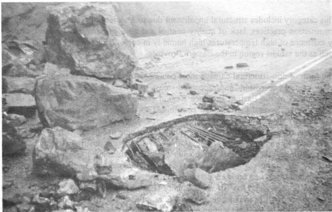
Plate 2. Slope slides-damaged bridge near Al-Baha region
