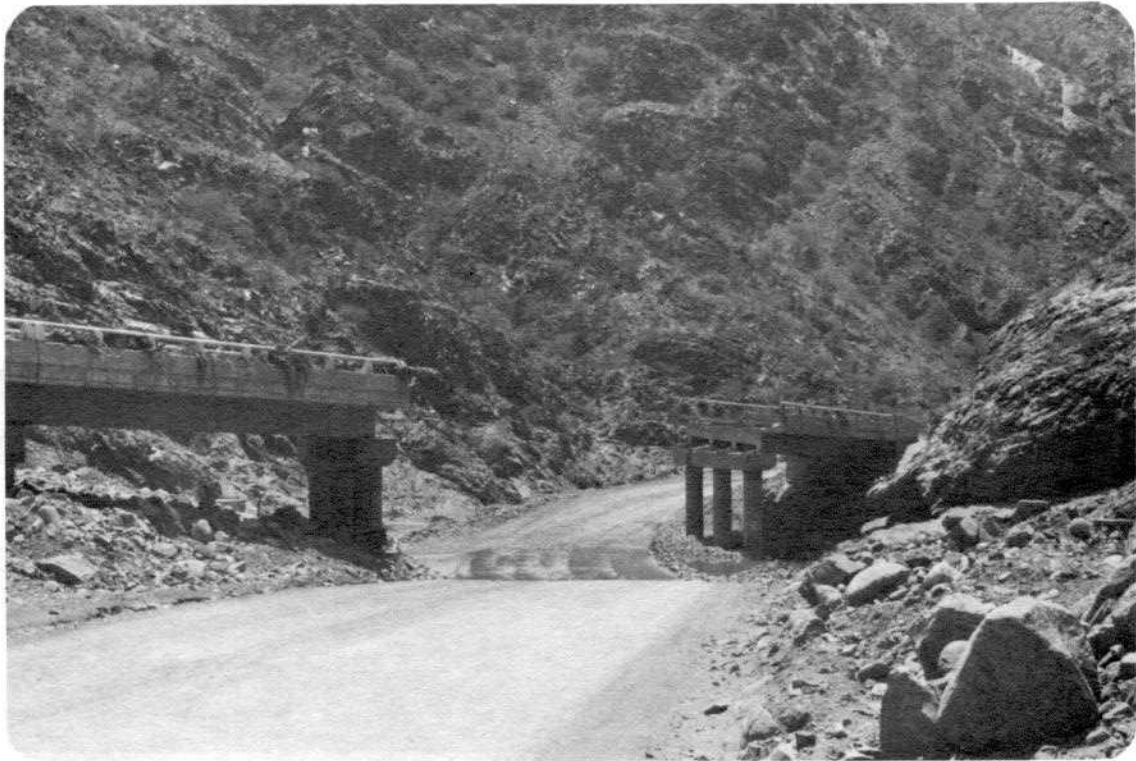
Plate 1. Flood-damaged bridge in Asir region
