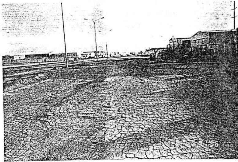
Fig. 2. Typical deterioration of pavements when calcareous bases are used in areas with shallow groundwater table
