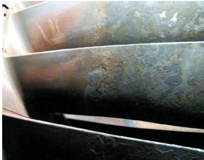
Fig. 11. Blades deterioration due to corrosion [27]
