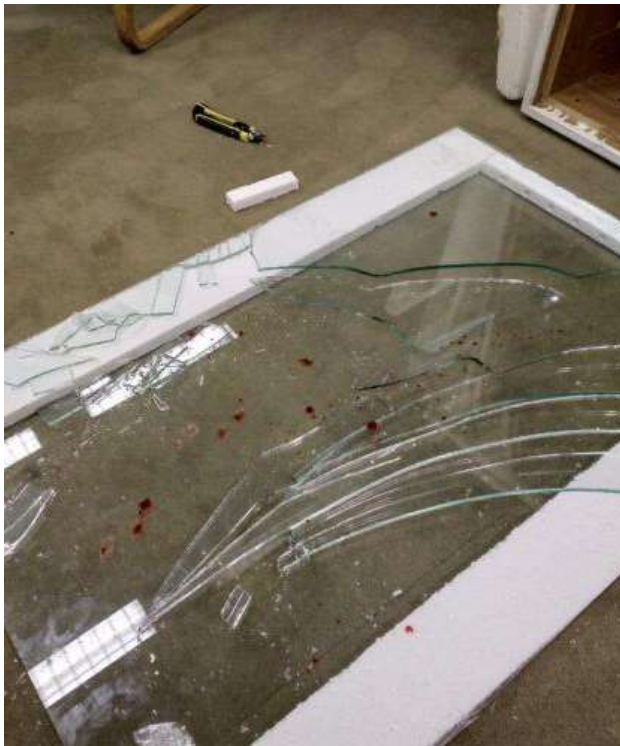
Failed trails- Glass structural failure
