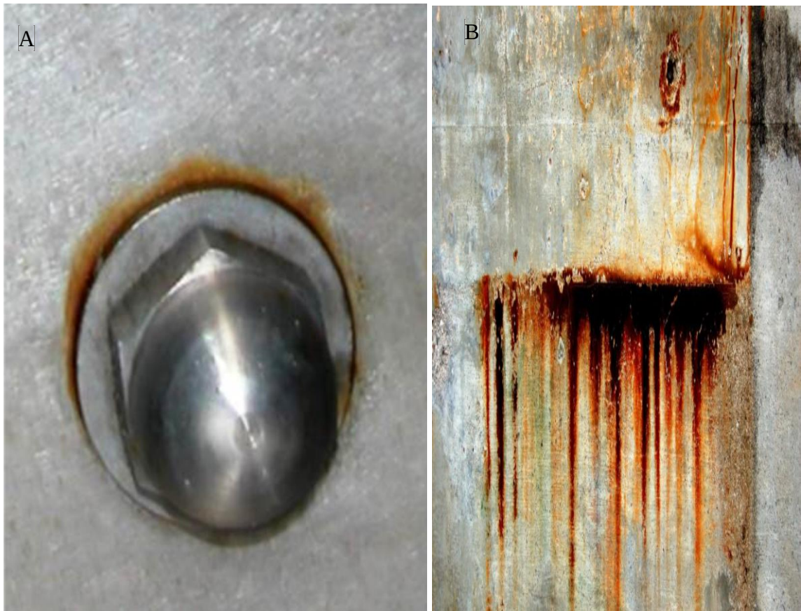
Fig. 1.6A & 1.6B Metal Crevice corrosion[26]
