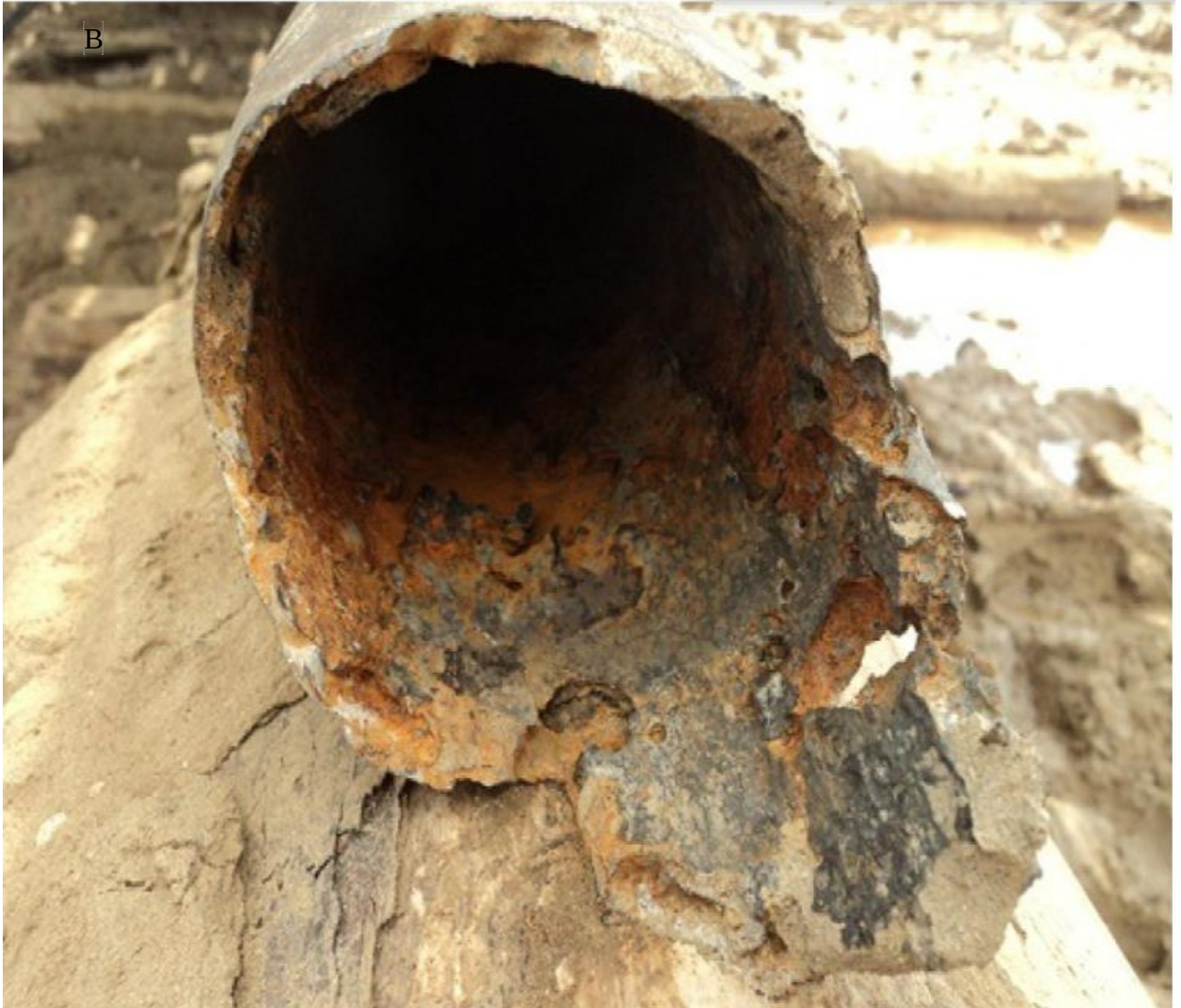
Fig. 1.4A & 1.4B Corrosion caused by H_2S [24].
