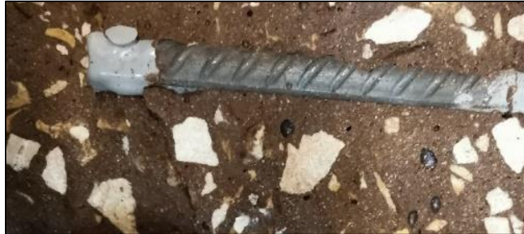
Figure 6-13 Rebar condition in a typical specimen after 360 days of exposure to 5% NaCl
