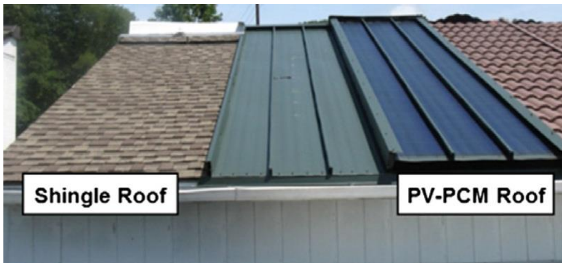
Figure 2.25 PV-PCM system installed on a naturally ventilated roof (taken from Ref. [52]).
