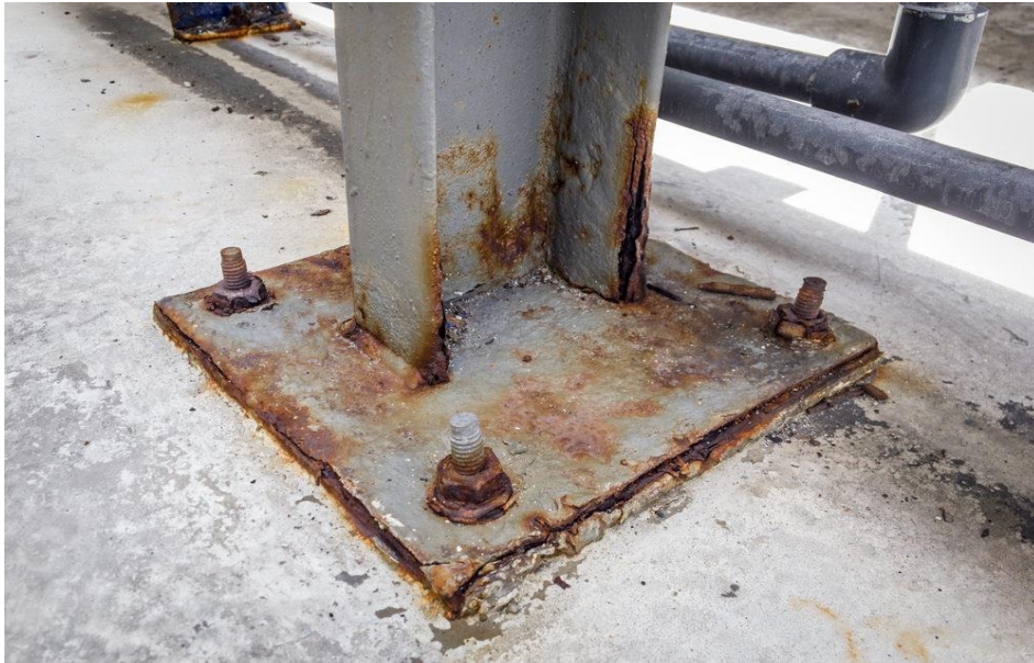
Figure 4: the surface of stainless steel showing clear signs of crevice corrosion.
