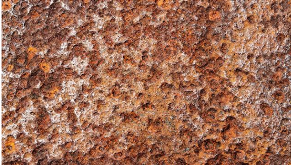
Figure 2: the surface of stainless steel showing clear signs of pitting corrosion.
