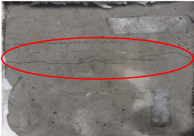
Figure 4. 21: Crack appearance of 0.35mA/cm 2 Specimen
