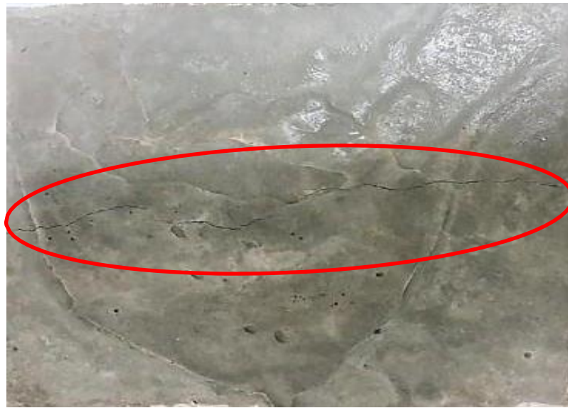
Figure 4. 26: Crack appearance of 0.40mA/cm 2 Specimen
