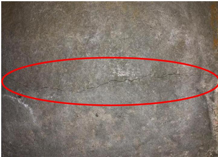
Figure 4. 6: Crack appearance on 0.20mA/cm 2 Specimen
