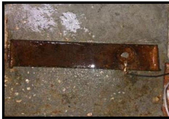
Figure 3. 13: Cathodic protection of embedded steel bar result counter electrode corrosion.
