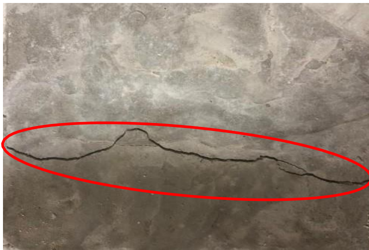
Figure 4. 16: Crack appearance of 0.30mA/cm 2 Specimen
