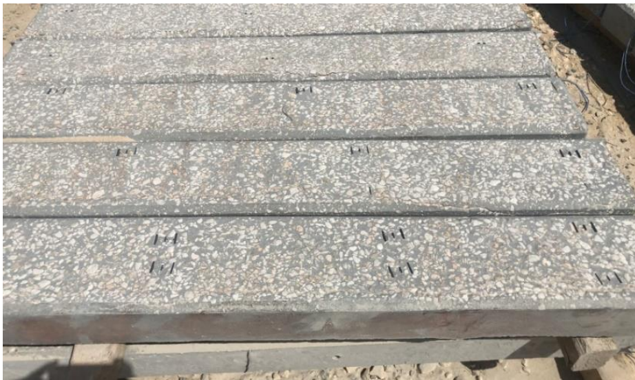
Figure 3.22: Sandblasted beams (after reinforcement corrosion process)
