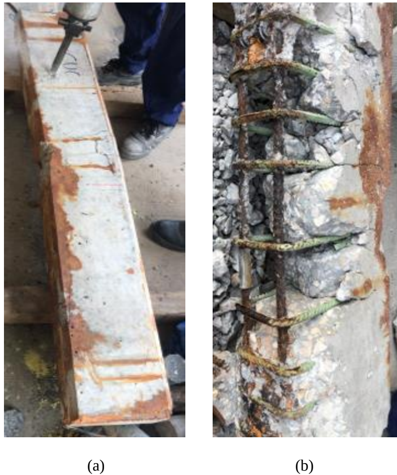
Figure 3.29: Extracting of corroded bars (a) Remove the concrete cover (b) Remove the surrounding concrete from the bars.
