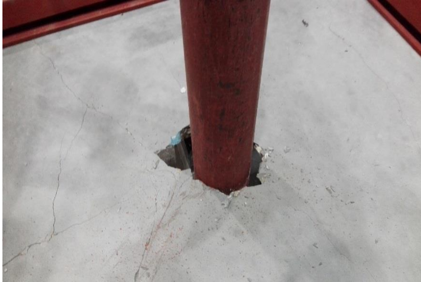
Figure 5.9: The impactor penetrates through the normal concrete slab
