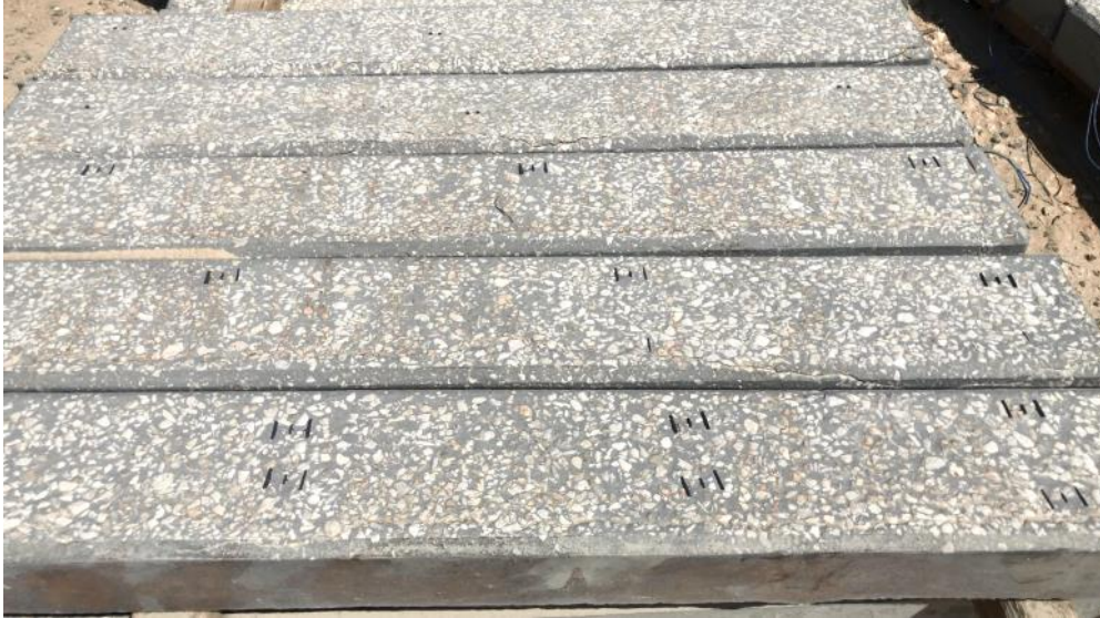
Figure 38: Sandblasted beams (after corrosion)
