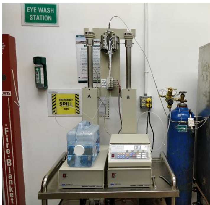
Figure 6. 6 Positive displacement pump
