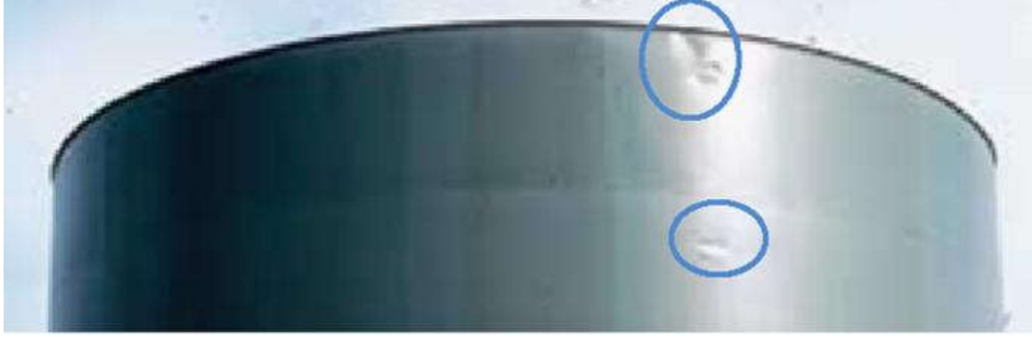
Figure 44 A tank with local damage [84]
