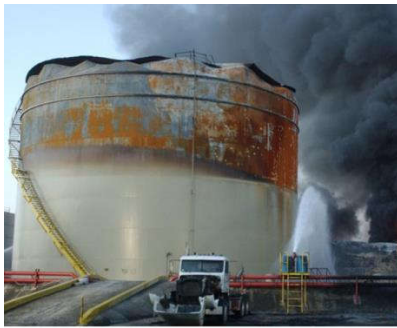
a) Buckling of a tank due to fire
