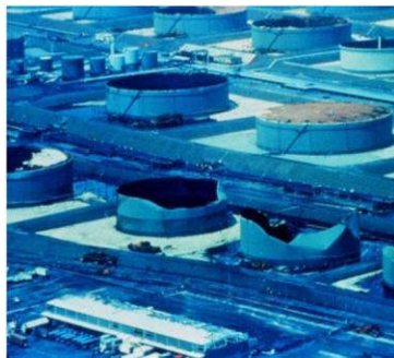
b) Buckling of a tank due to wind load
