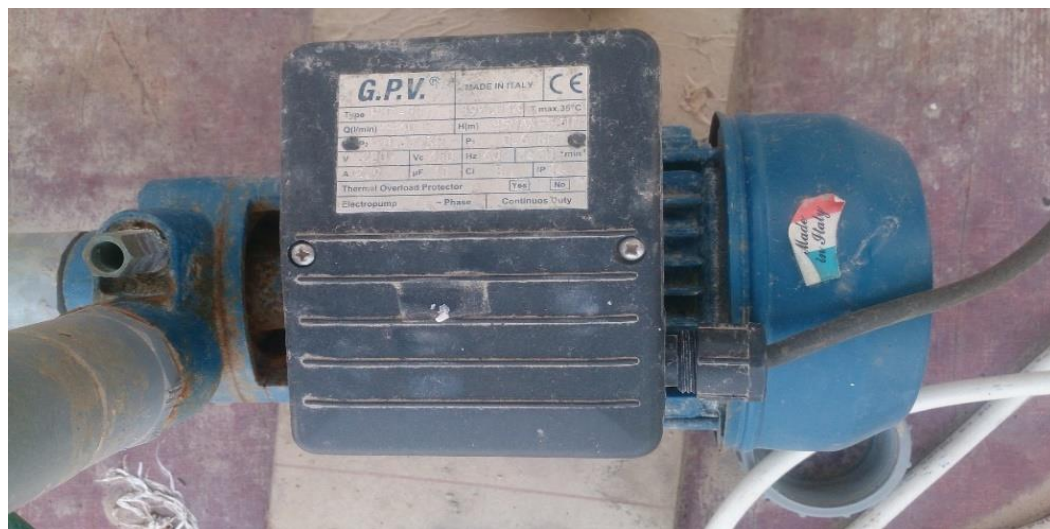
Figure 2.6: The electric water pump
