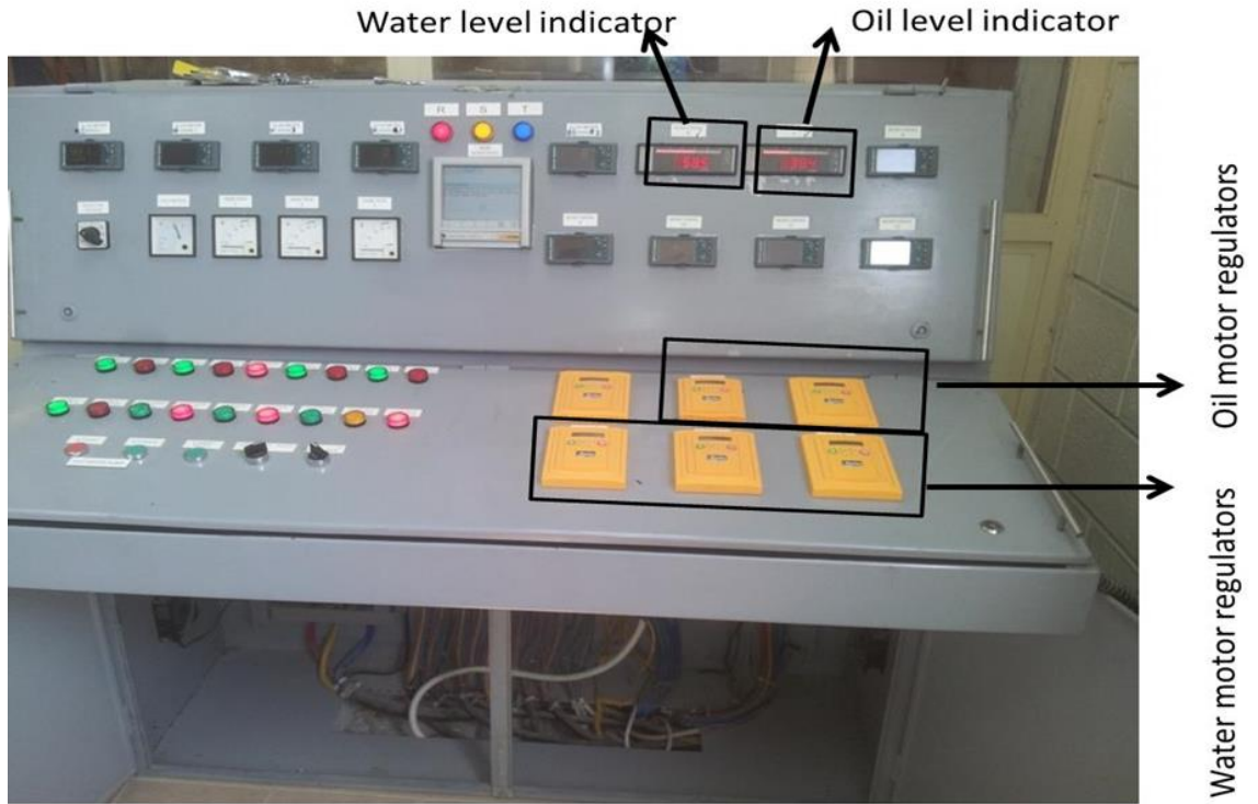
Figure 3.7:-Photograph of control panel of multiphase flow loop
