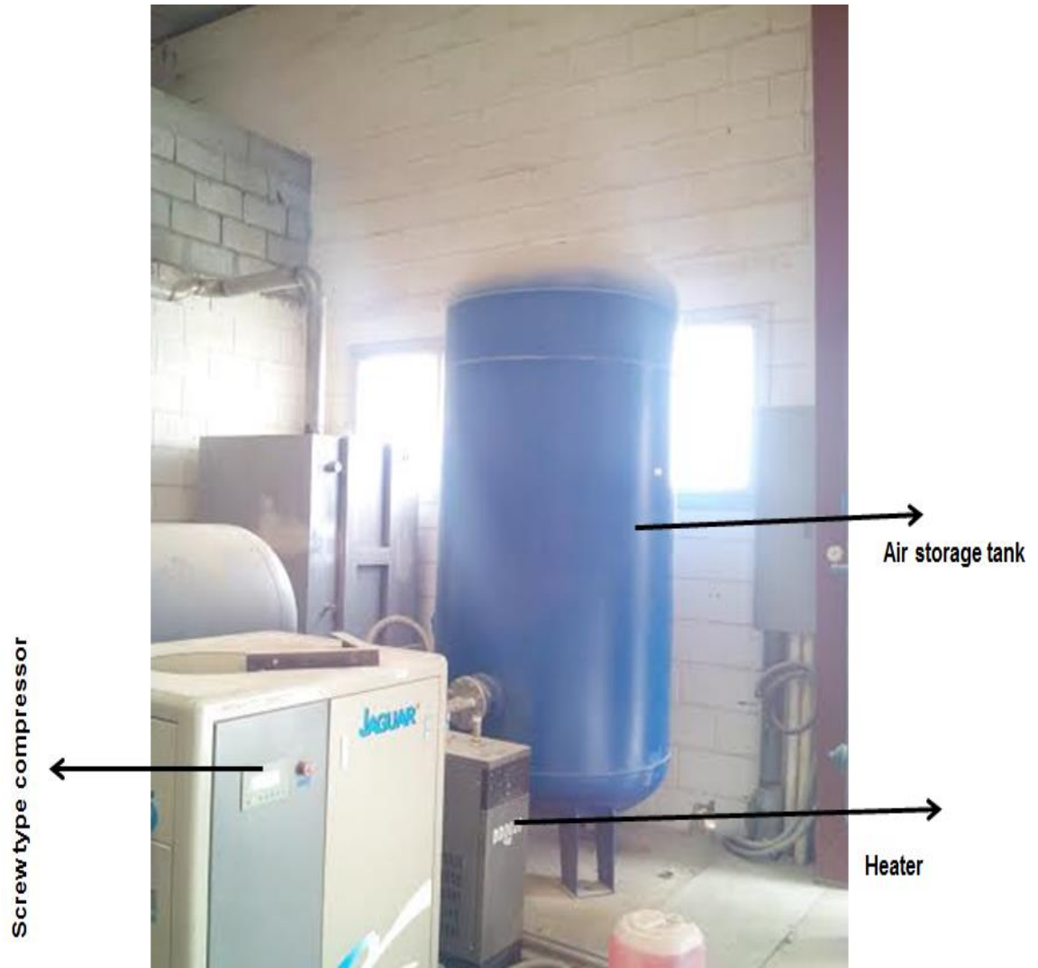
Figure 3.6:- Photograph of compressed air system.
