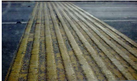
Figure 1.3: Short periodic humps at Tanajib/ Safaniyah main road intersection.
